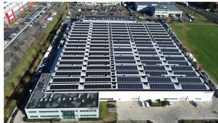
Walvoil – Photovoltaic plants on factory roof in Castel San Pietro (Italy)
